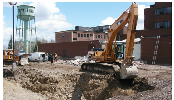
In April 2002, work was well underway on the north end of the property as RMH began to double in size with an expanded Emergency Department, a Mental Health Unit, Palliative Care and Continuing Care wing.
